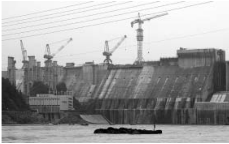
Danjiangkou dam in China's Hubei province is under construction for the middle route of the South-to-North project to relieve water shortages in northern areas.
