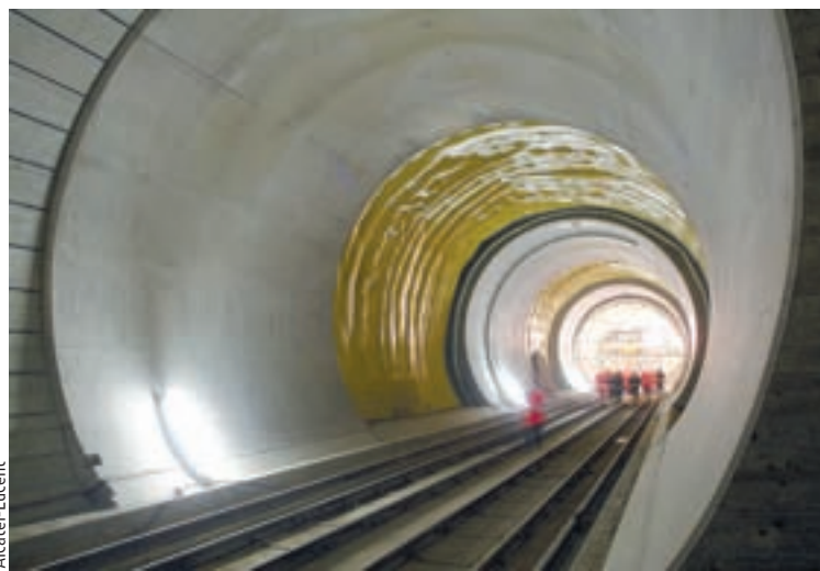
The Gotthard Tunnel is being constructed under the Alps between Switzerland and Italy.
