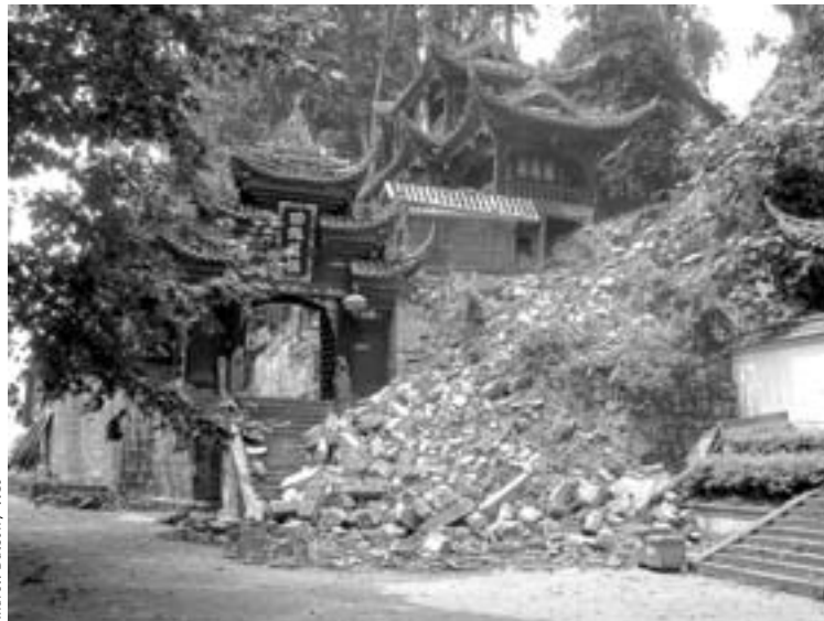
Reconstruction of the quake-damaged Erwang temple will be part of the plan to revive the Dujiangyan tourist industry.
