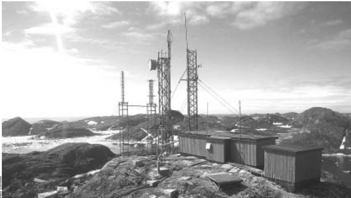
Nav Canada has installed ADS-B receiving antennas in Greenland to receive flight information from trans-Atlantic airline flights. The system will be expanded next year, providing coverage over much of the Atlantic Ocean.
