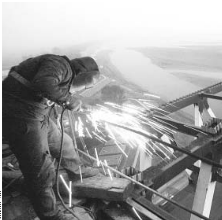
A welder works Thursday on construction of a bridge in Zhengzhou, China.
