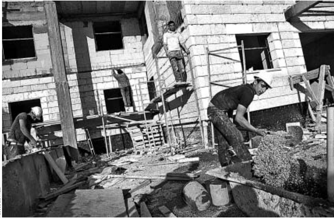
Palestinian construction workers at work at a housing development in the Jewish neighborhood of Har Homa in Jerusalem Monday.
