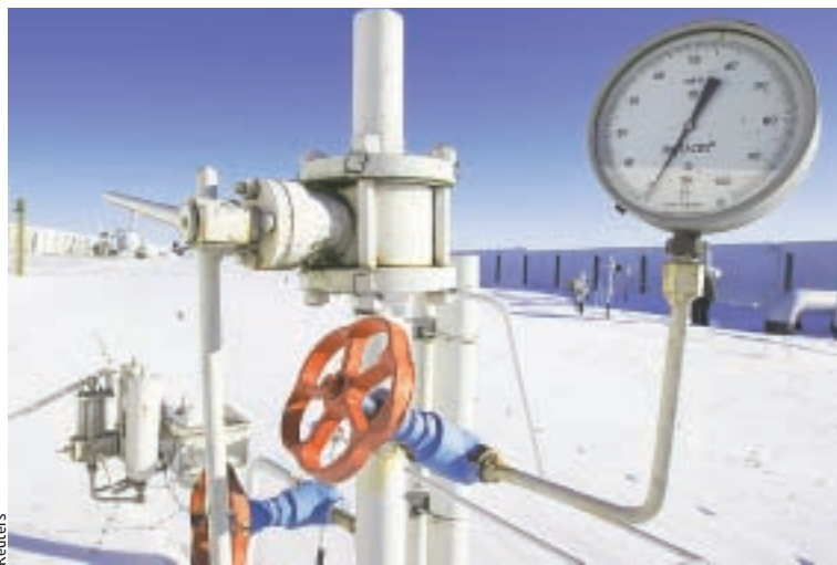
The arrow of a pressure gauge points to zero at a Ukrainian gas compressor station in the village of Boyarka after Russia shut off natural-gas supplies.
