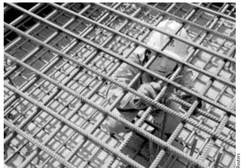
A worker installs steel bars in Shanxi province Tuesday. Steel has been the backbone of China's growth and pricing for state mills is a key government concern.
