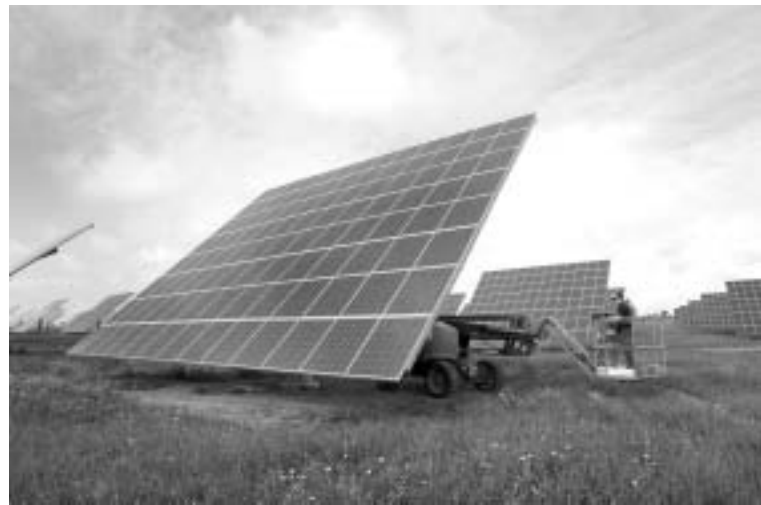
Acciona's profit rose sharply on gains related to the sale of its Endesa stake. Pictured, a technician inspects a solar panel at the company's power station in Portugal.
