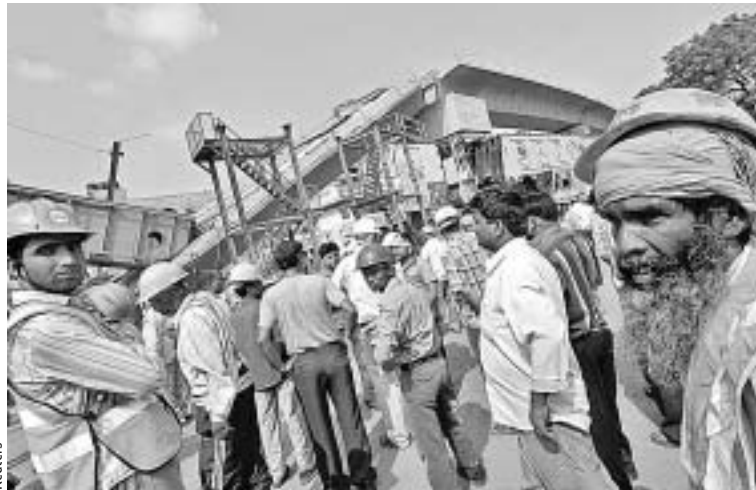
Workers and rescuers stand at the site of a collapsed Delhi Metro bridge in New Delhi this month. Metro builder Gammon India faces possible blacklisting.
