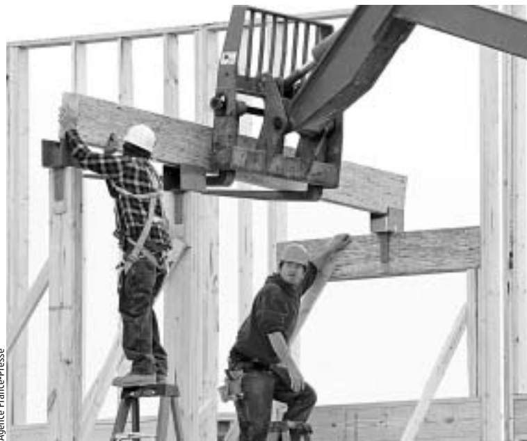
Construction workers lift beams into place on a structure in Manassas, Va. Upbeat housing data were offset by another grim report on the state of U.S. manufacturing.
