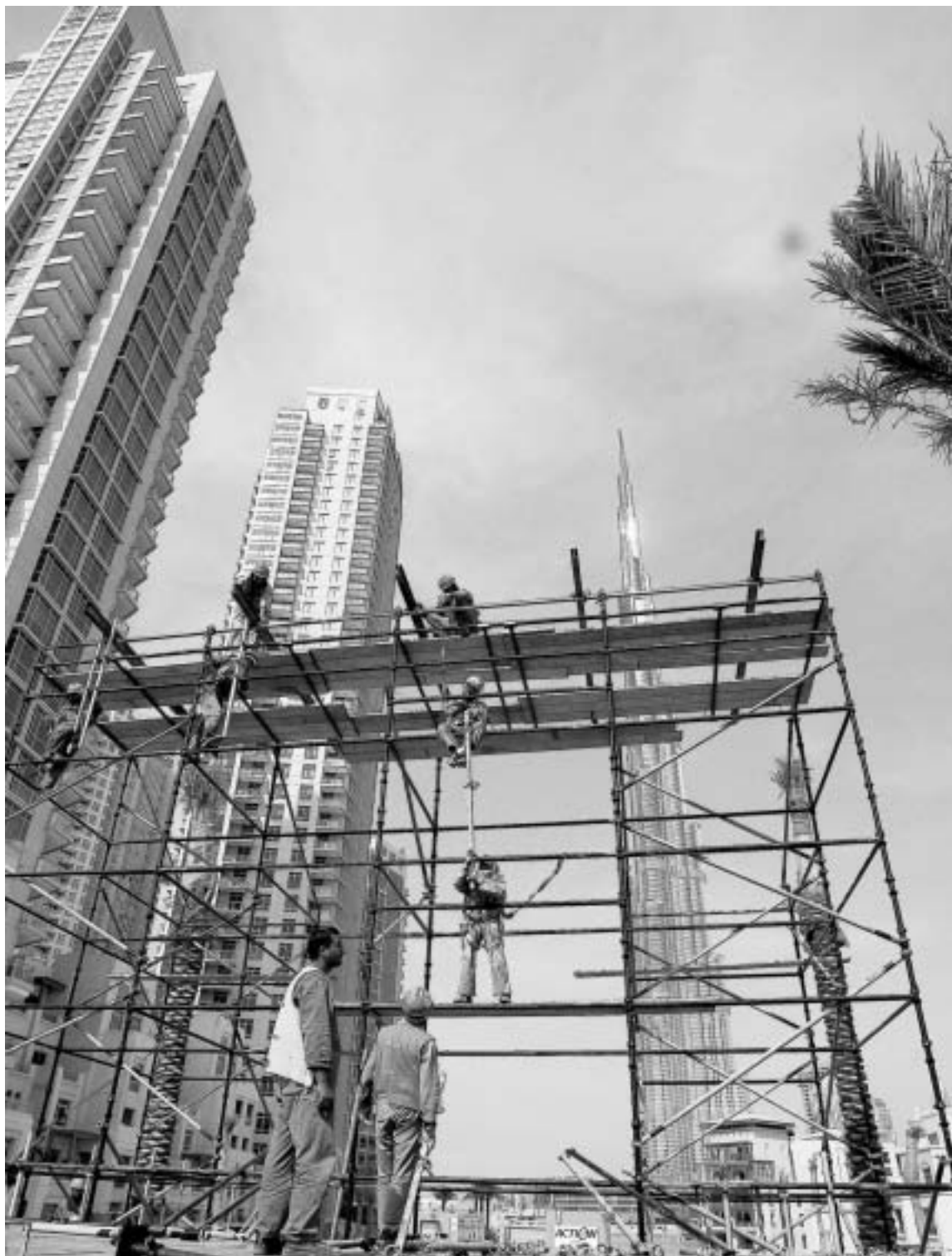
Workers at a construction site near the Burj Dubai, which, at 800 meters, is scheduled to open in January as the world's tallest building.
