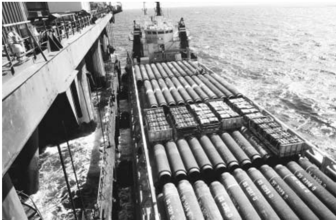
A barge holds sections of pipe in a handout photo from Nord Stream, which plans to build a gas pipeline under the Baltic Sea.
