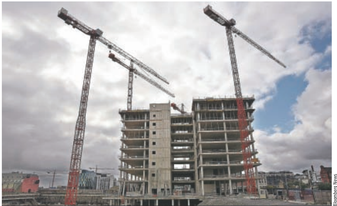
An unfinished commercial-building site in Dublin. Ireland's exporters are now sharing the pain of the construction sector.
