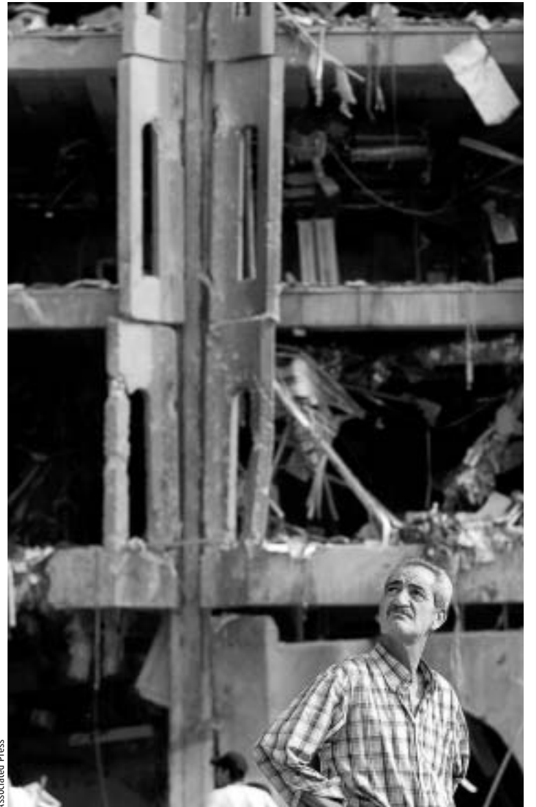
A man stands before the destroyed Ministry of Justice in Baghdad on Thursday. The building was hit by a bombing Sunday in which 155 people were killed.
