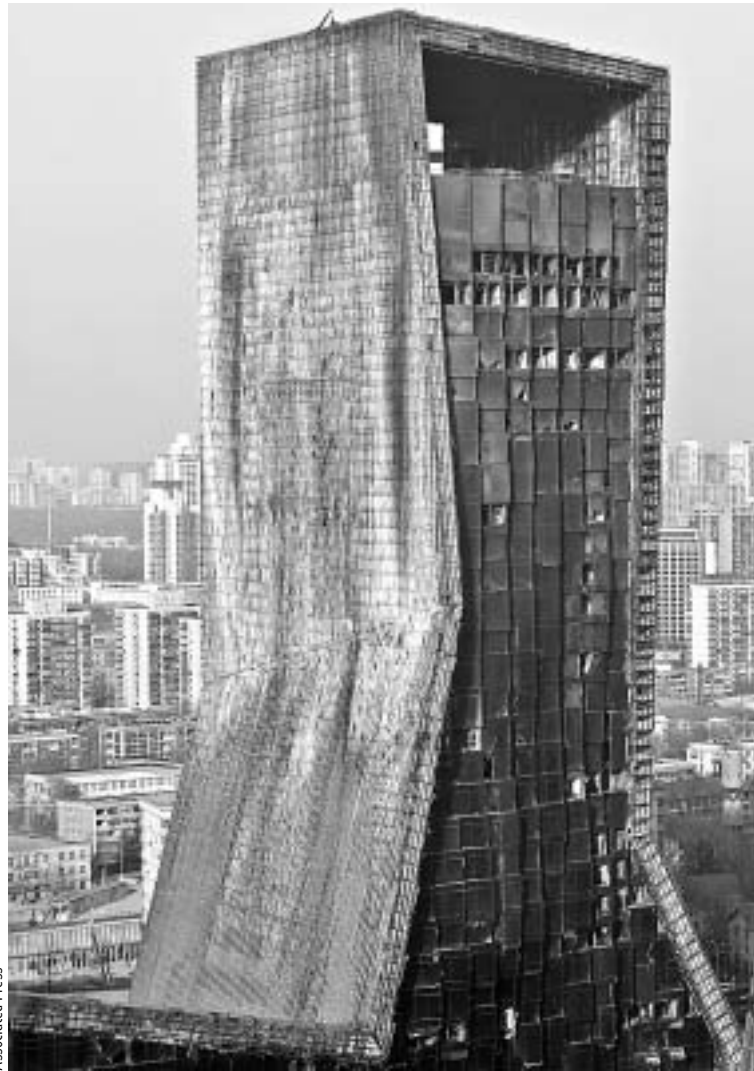
Part of the damaged building in state broadcaster CCTV's compound in Beijing on Tuesday. The fire was attributed to an employee-organized fireworks show.
