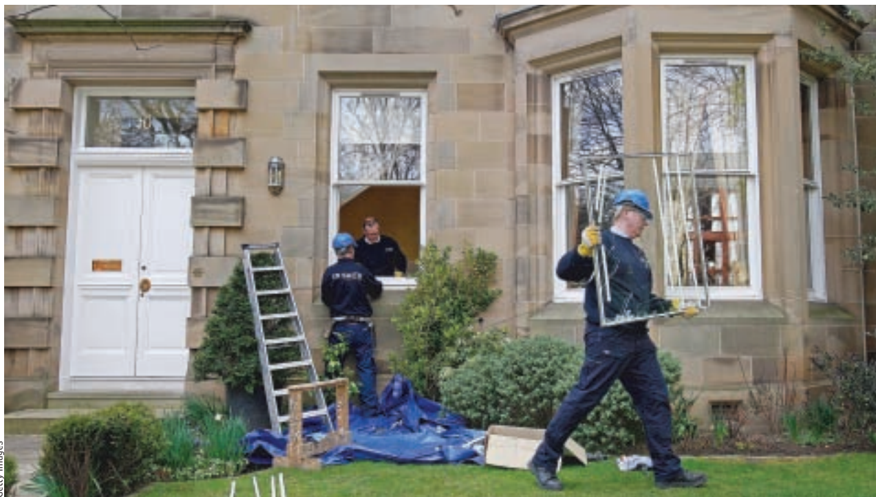
SHATTERED: A glazier removes a broken window after vandals attacked CEO Sir Fred Goodwin's Edinburgh residence. Page 2.
