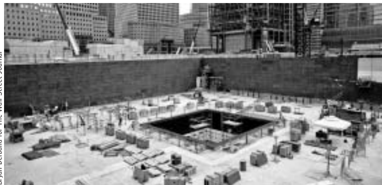
Work on a reflecting pond at the 9/11 memorial of the World Trade Center site.
