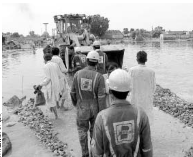
Workers repair a road damaged by the flood in Punjab province on Tuesday.
