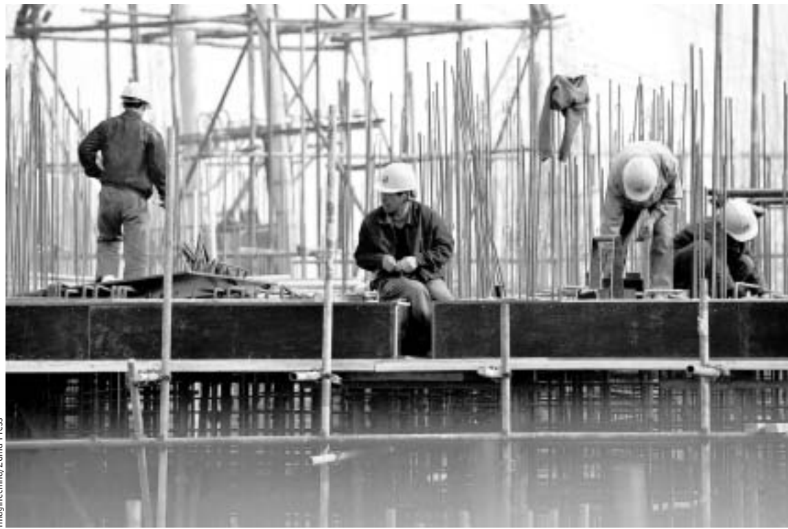
A construction site in Shenyang, above, in northeast China's Liaoning province, where Vice Premier Li Keqiang, right, was Communist Party secretary.
