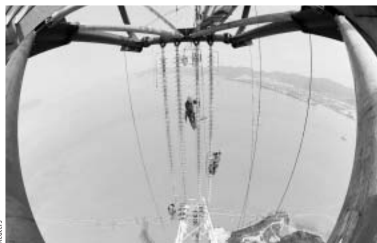
China says it isn't the world's largest consumer of energy. Above, workers install insulators on electric pylons in Hangzhou, Zhejiang province.
