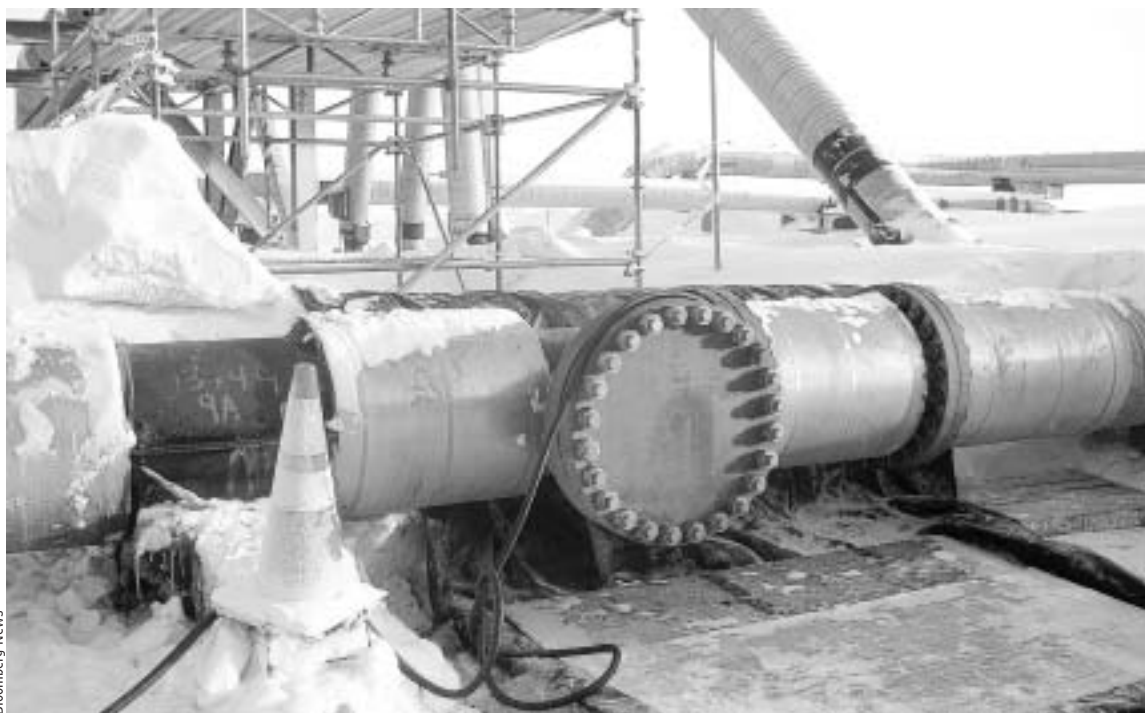
A section of a BP oil pipeline near Prudhoe Bay, Alaska, pictured in February 2009.
