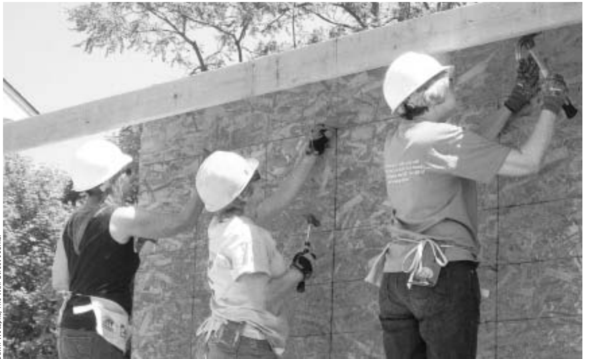
Habitat for Humanity volunteers help build the home of Cheri Sabolenko in East Patchogue, N.Y., in May. The charity's closings fell 3% last year, when other builders saw far steeper drops.
