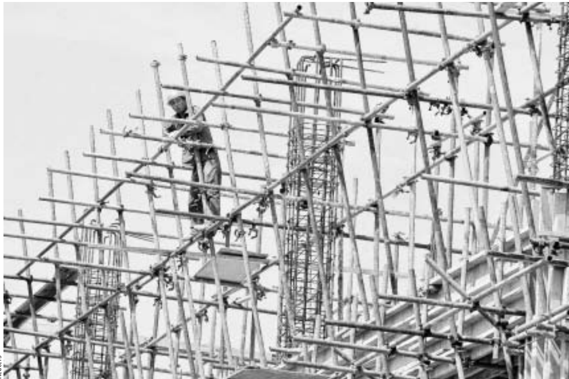
A construction site in Nanjing, China. A property boom helped fuel surprisingly rapid growth in the first quarter.
