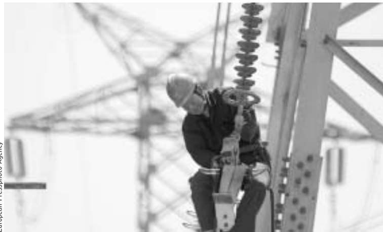
A worker sets up power lines on a high-voltage electricity tower in Qingdao, a city in eastern China's Shandong province, in May.
