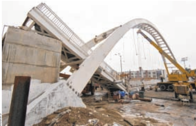
A footbridge to Jawaharlal Nehru Stadium in New Delhi collapsed Tuesday, injuring workers and adding to setbacks before the Commonwealth Games.
